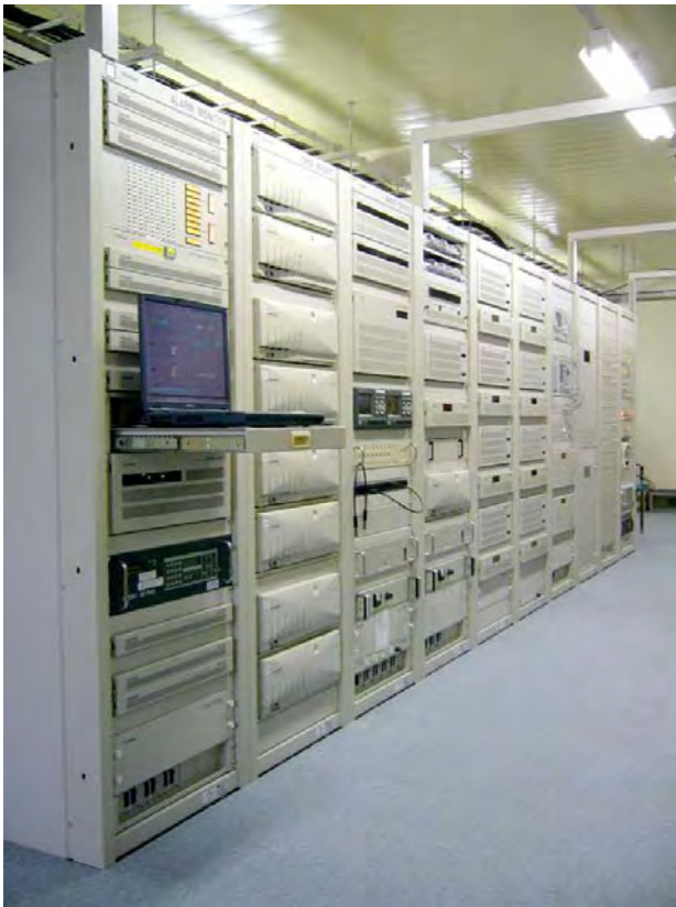
Rack room of master control
