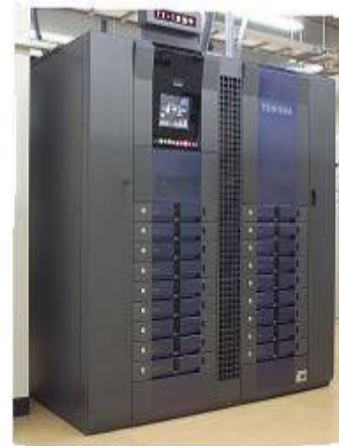
3 kW digital transmitter rack
